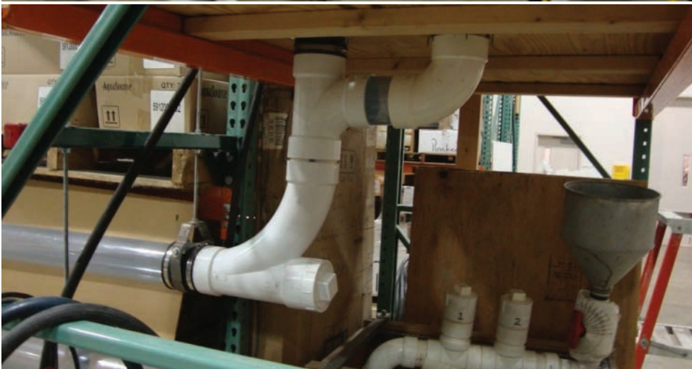
PHOTO 4-E PLUMBING UNDER FLUSH STAND
